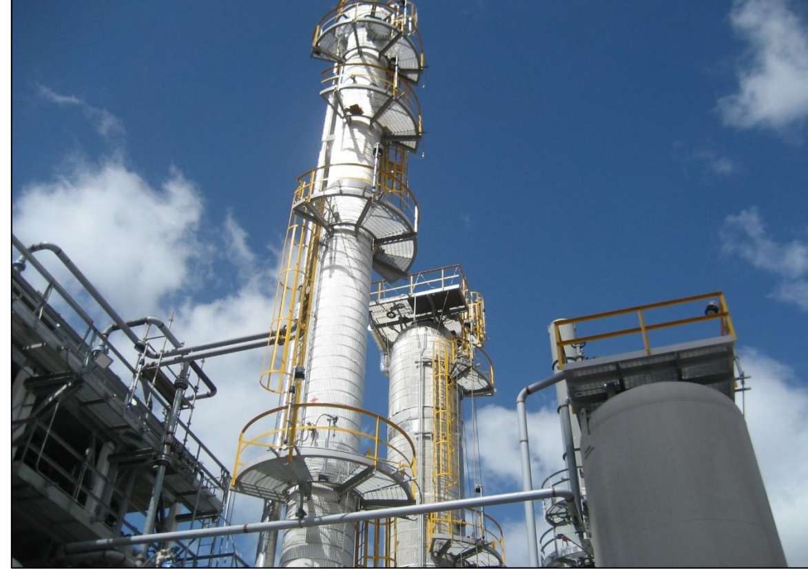
Hydrotreater Unit for Renewable Fuels
