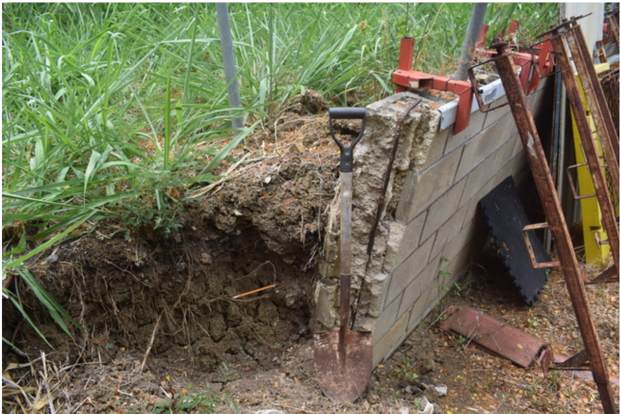
Photo 1 caption: This 5-foot high, permitted CMU retaining wall failed in March after substantial rains. The wall runs parallel to the drainage easement along our mauka property boundary, about 7 feet from the concrete-lined drainage ditch. Even with that close proximity to the ditch, note the occurrence of large shrink-swell cracks in the soil; these are evidence of considerable subsurface water flow during wet periods.
